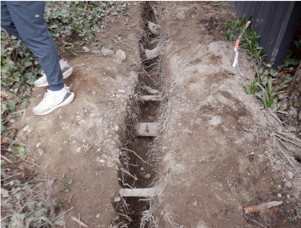
Cluster of structural roots exposed west of Trees C & D
