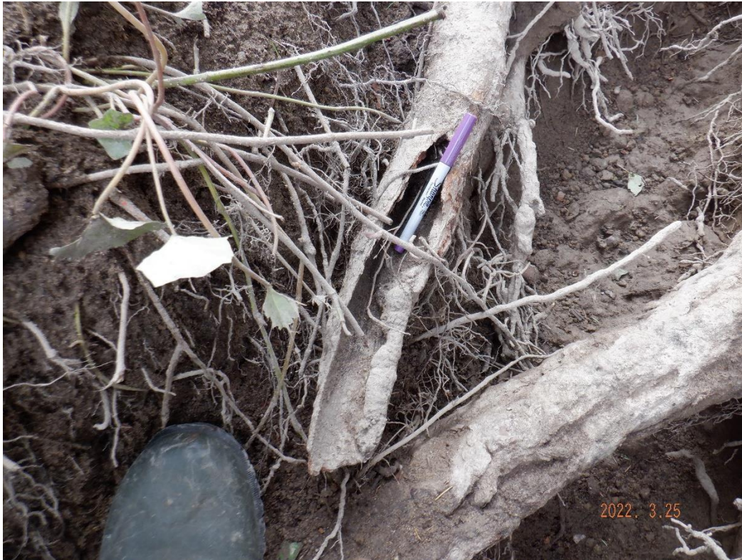
Decayed root pictured above at edge of proposed footing, can be pruned away
